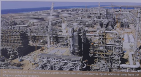
Our Petro Rabigh joint venture integrates a petrochemical plant with a refinery to capture additional value from the Kingdom's petroleum resources.
