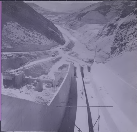
Water spillway and hydro-electric power generating station.
