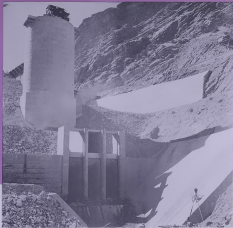
Front of the concrete Dam. The main intake can be seen with its three steel gates and control tower.
