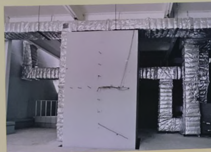
Thermal Storage and Ducting for Air System
