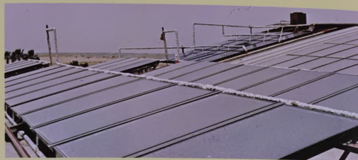
Water and Air Solar Collector Array
