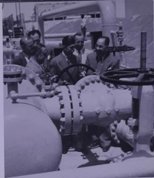
Left: The Baij-Baghdad 12-inch pipeline feeding the Government refinery at Daura was commissioned in April 1955. H.E. the Minister of Economics, Dr Nadin Pachachi, is in the centre of a group of distinguished visitors
