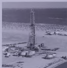
Crew prepares to pump drilling mud at this Manifa well. Most Manifa wells are offshore in the Gulf.
