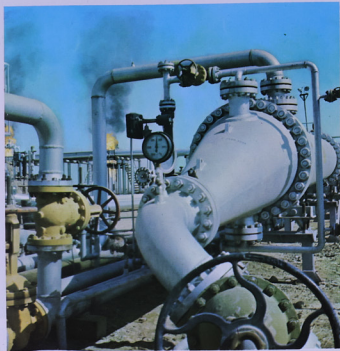
Gas-oil separator unit at Marun.
