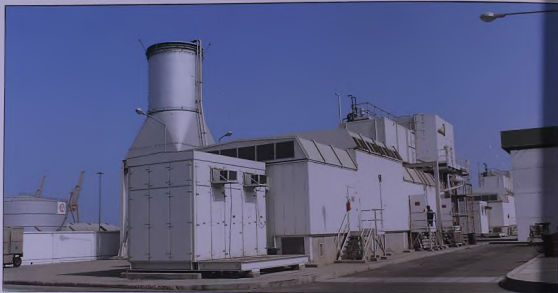
Gas Turbine " C " - Layyah Station
