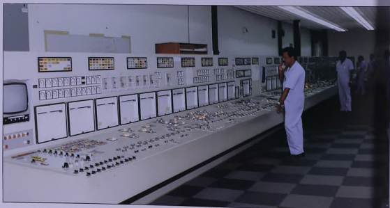
Phase II & III Units Control Desk
