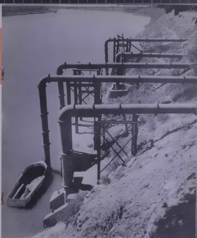
A number of big pumping engines on the River Tigris.
