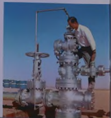
H. P. Walter checks a water-supply well, part of Abqaiq injection system.
