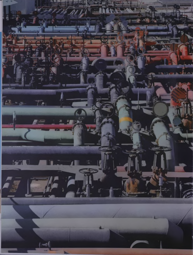
Special colors are employed to identify the many pipes at Aramco's Ras Tanura terminal.
