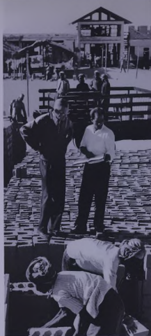
A Dammam plant manufactures cement blocks for the construction of loan plan houses there.
