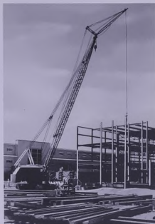
Aramco's new administration building, adjoining the existing one, will centralize Dhahran offices.
