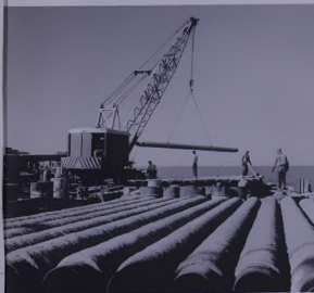
Steel pipe from nondollar sources is concrete-coated for underwater part of Safaniya pipeline.
