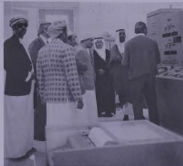
The visitors are shown over the control room of the Main Line Pumping Station in Fahud by Senior Production Supervisor, Tom Parea.
