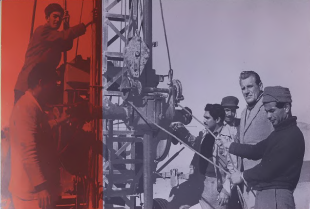
Water for Man and Beast, well drillers at work in the desert.
