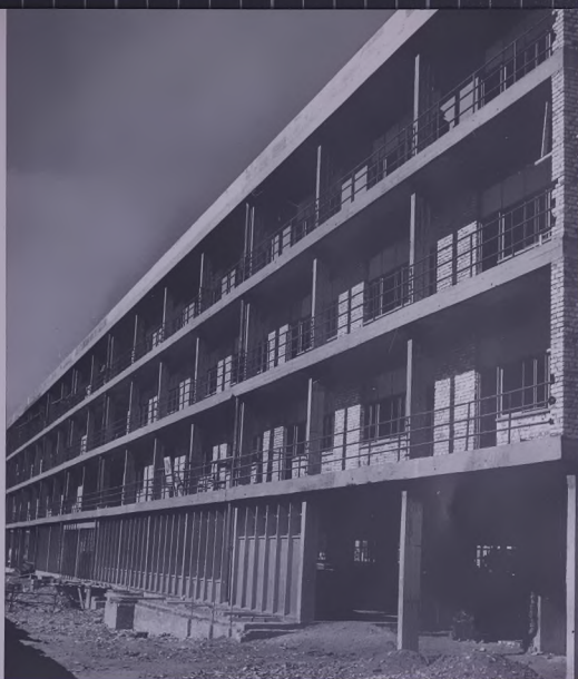
Students' hostel under construction in Baghdad. There has been an immense increase in the number of students in institutions of higher education.
