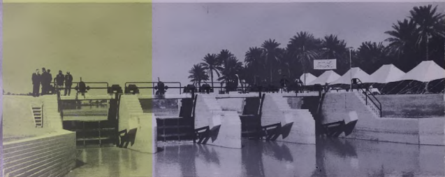
Regulator on the Mussayib Irrigation Canal; part of the elaborate system by which water levels are controlled.
