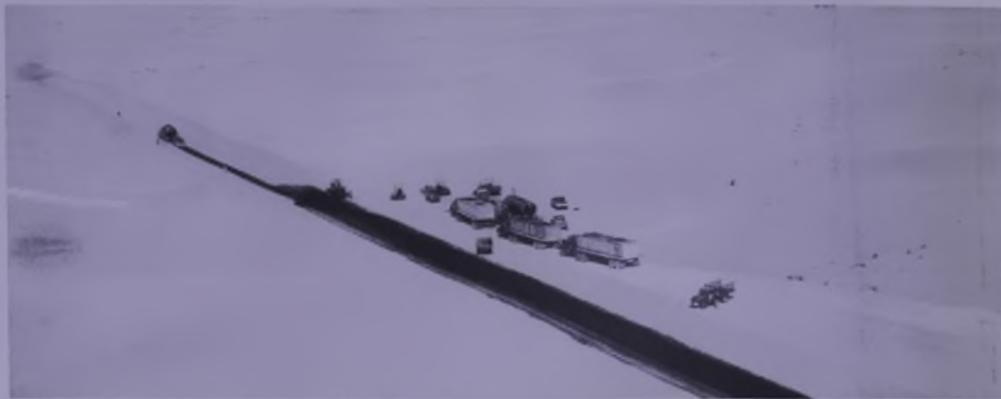
A road being built northward from Qatif will give quicker access to the Safaniya and Manifa Fields. Aramco has built many roads necessary for its operations which also are used heavily by the public.
