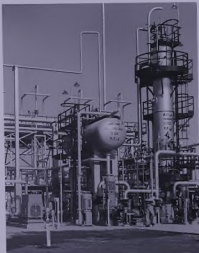
New liquefied petroleum gas processing units in Alzabir, a part of expanded facilities that increased LP Gas productive capacity to 12,000 barrels daily.
