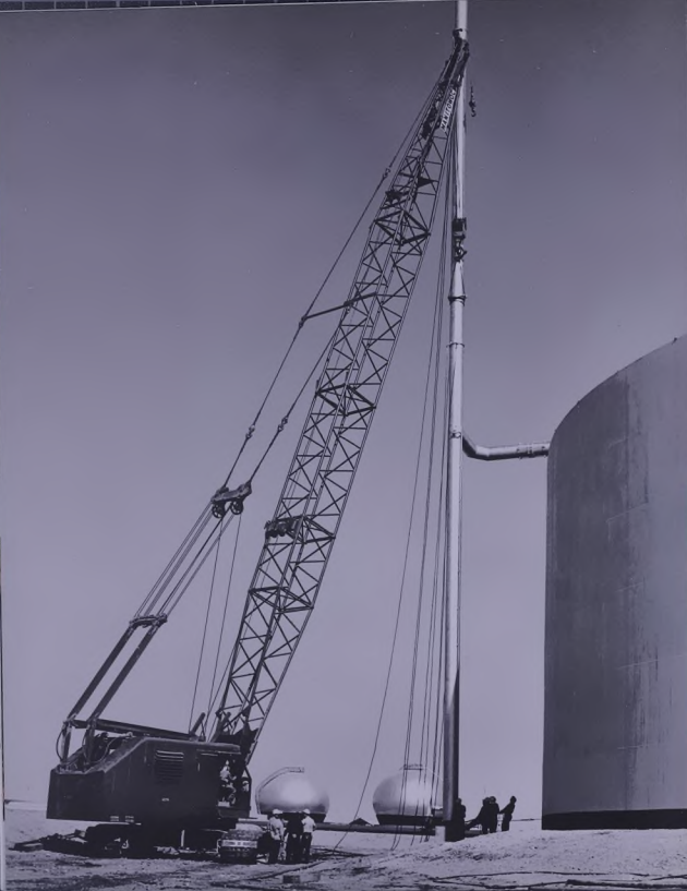
A gas vent pipe is joined to a newly built crude oil storage tank near Abqaiq.
