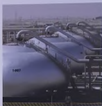
The company's gas facilities supply an increasing stream of natural gas to the Kingdom's Master Gas System. Opposite: An engineer checks a valve at Ju'aymah Gas Plant.
