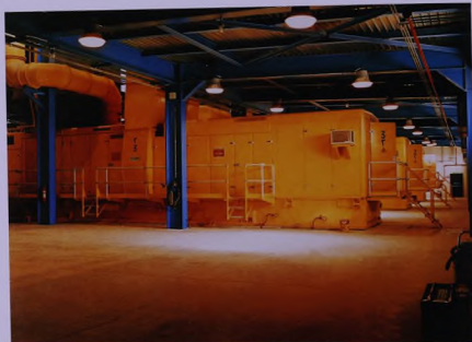
ARAR power plant. Saudi Arabia 3 gas turbines. General view inside the turbine building after 6000 hours of firing.
