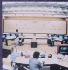
The control room. The entire plant is monitored and controlled from 3 workstations. Mimic panel in background.
