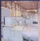
One of the two machine halls of Riyadh 8 power plant, with BBC Type 11 gas turbine sets.
