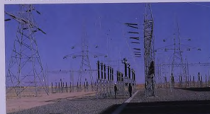
HAIL ELECTRIFICATION - 132 kV TERMINAL
