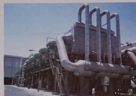
Sea Water Desalination Units at Sitra Power & Water Station.
