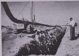
The construction of the gas line to take natural gas to Manama Power Station.
