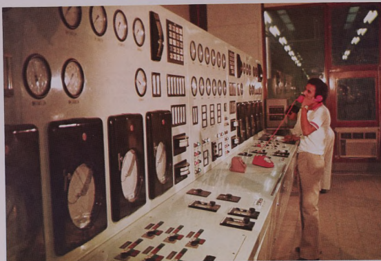
Thermal Control Room at Sitra Station.
