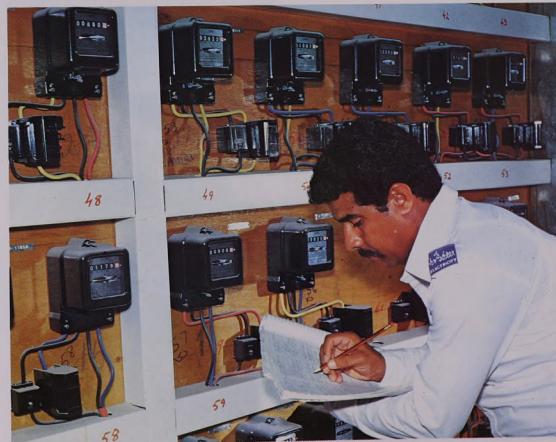
Electric Meter Reader.
