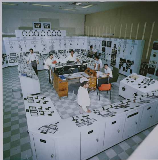
Control Room at Manama Power Station.
