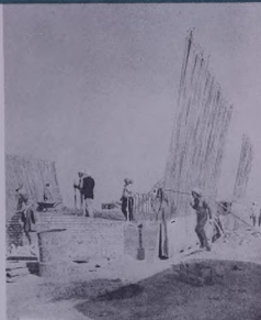
Construction work is seen being carried out on one of these bridges.
