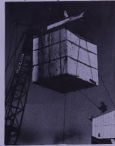
The switchgear had to be lowered through the roof of the power station.
