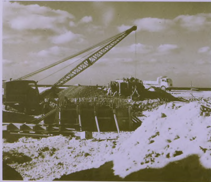
Work went on day and night to lay the foundations for the modern industrial complex
