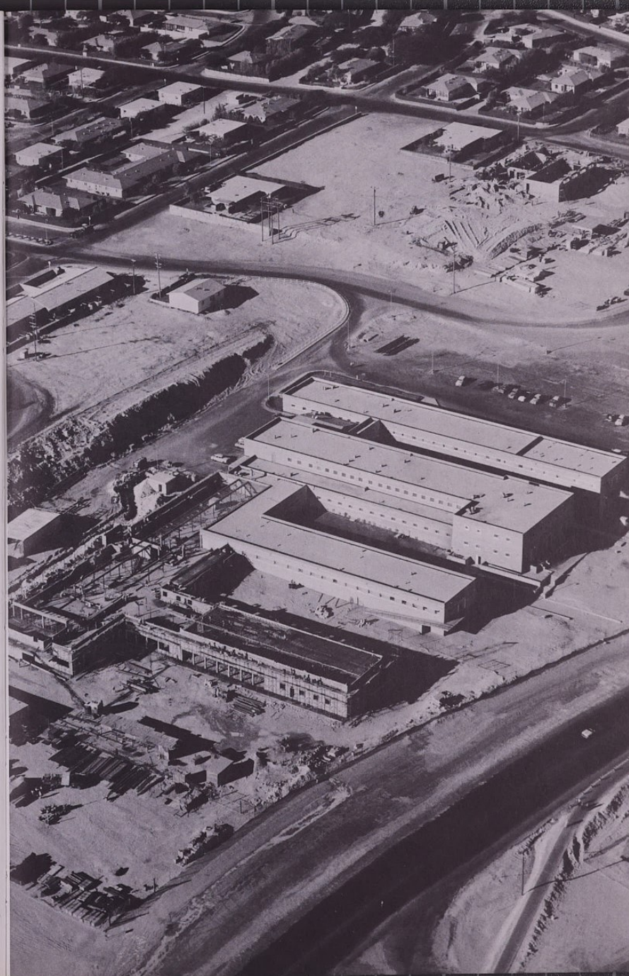
A new wing under construction at Dhahran Health Center will be completed in 1956.
