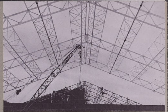
Steel girders are set in place for roof of a new storehouse.
