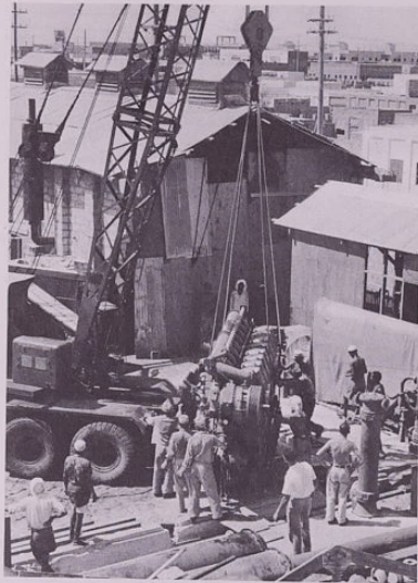
To meet a growing demand for electricity, the al-Khobar power plant increases its capacity by installing an additional 14-ton generator.
