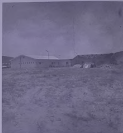
View of Mina al-Fahal Clinic showing new six bed extension being added to the main building.
