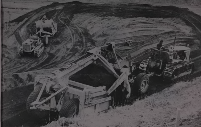
Grading machines pulled by tractors prepare a hair-pin curve on a steep section of a CENTO road project.
