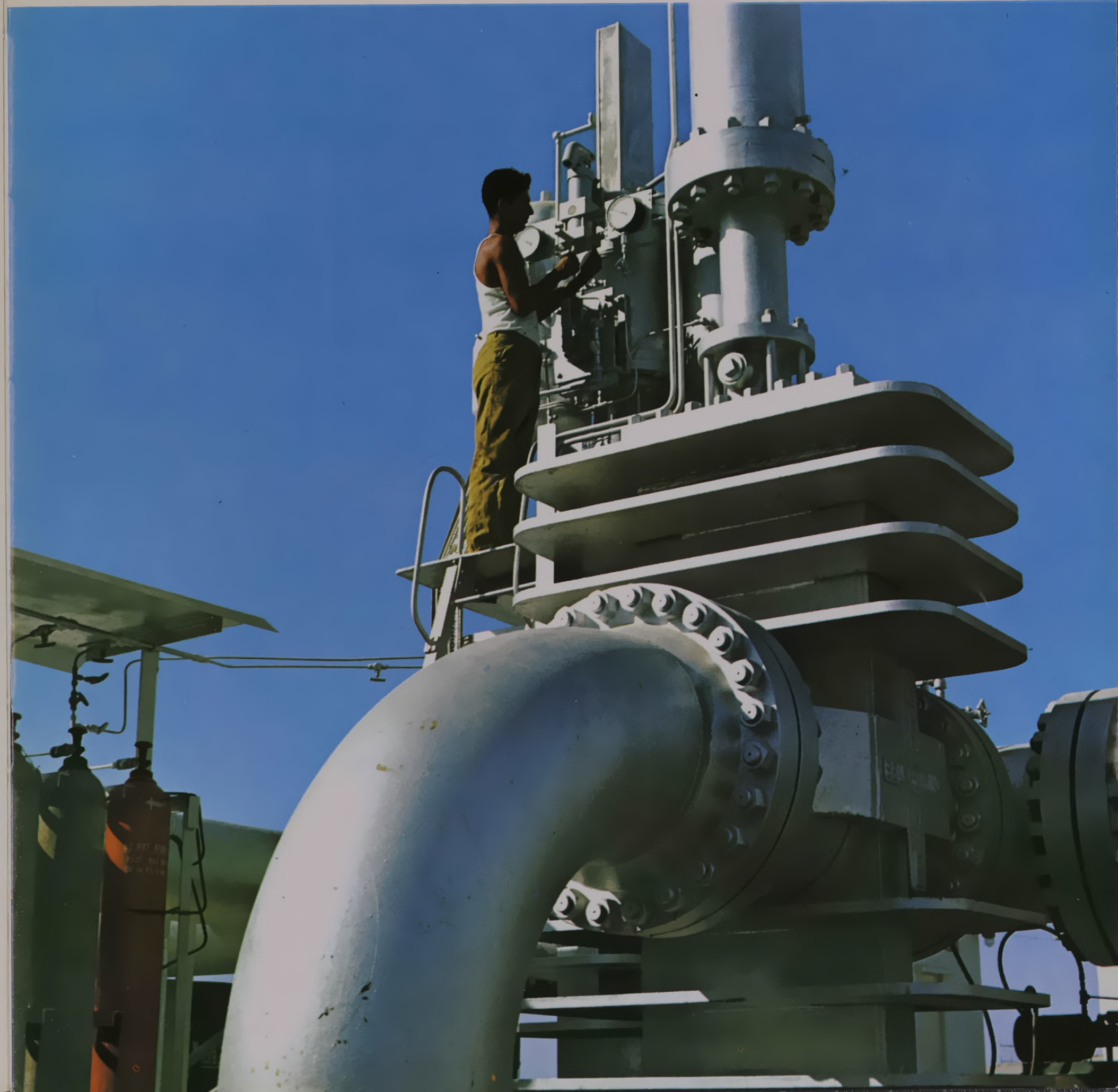
Main pipeline enters Mina al-Fahal tank farm
