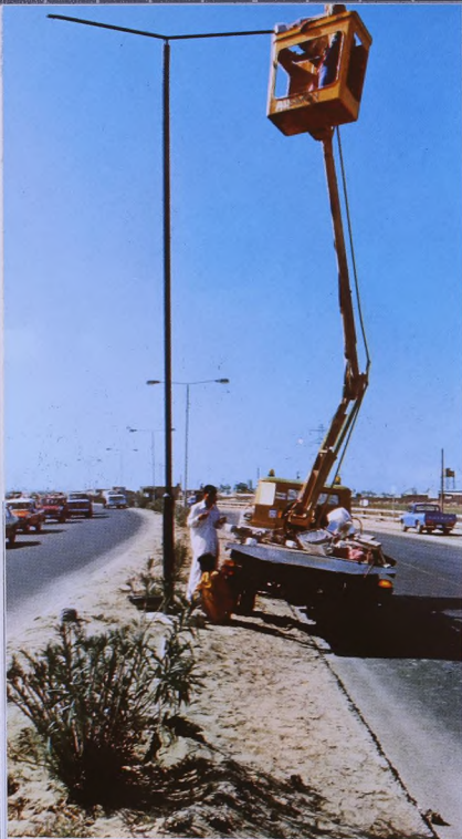
Street Lighting Section of the Directorate is responsible for installation and maintenance of street lighting in Bahrain
