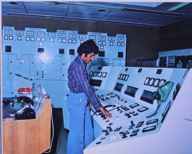
Operator increases turbine output in the Control Room at Sitra Power Station
