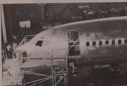
The plane completely stripped off of its paints
