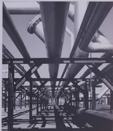
Complex of pipes leading from refinery unit.
