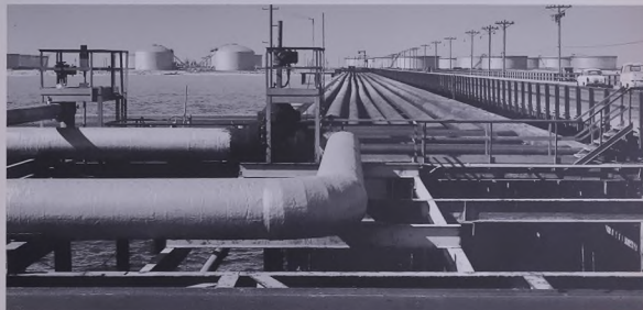
Heavily insulated pipelines carry refrigerated LPG from new plant (upper left) to tankers at north pier.
