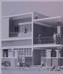
An employee home nears completion in Dammam, one of more than 3,300 acquired under the program.
