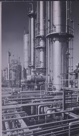
Operator visually inspects alkylation plant.
