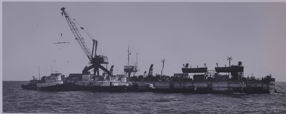
Pipe-laying barge puts down lines that help increase Safaniya field capacity to 325,000 barrels daily.
