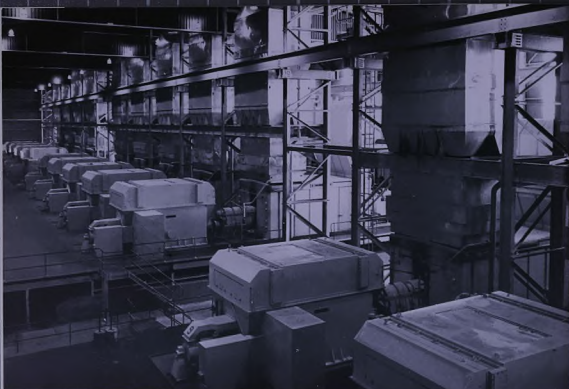
Part of the turbine hall having eleven of the eighteen turbine generating sets. The power station is the largest gas turbine generating station in the world and when completed will have a total installed capacity of almost 300 MW.
