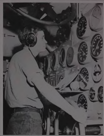
During precision-like manoeuvres, engine room crews maintained an alert watch over the operation of powerful, but delicate propulsion machinery.
