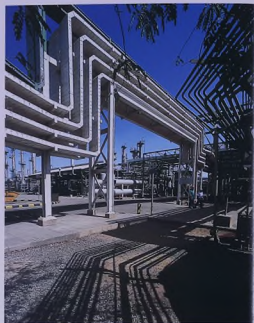
Pipes zigzag at Riyadh Refinery.
