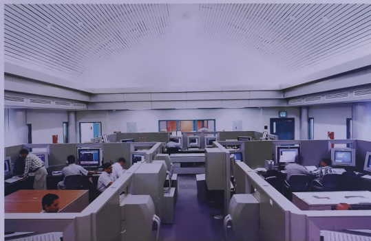
This control room at Abqaiq Plants will soon benefit from a new process data networking technology.
