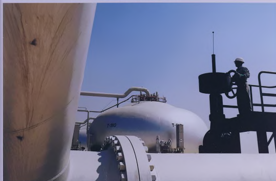
A spheroid, center, at Abqaiq Plants holds associated gas released from crude oil.
