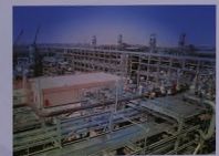
Distributing energy to the world requires a massive processing and distribution network. A portion of the massive Hudeybah Gas Program, completed this year, is shown during construction.
