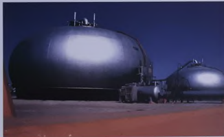
Part of the Master Gas System.
