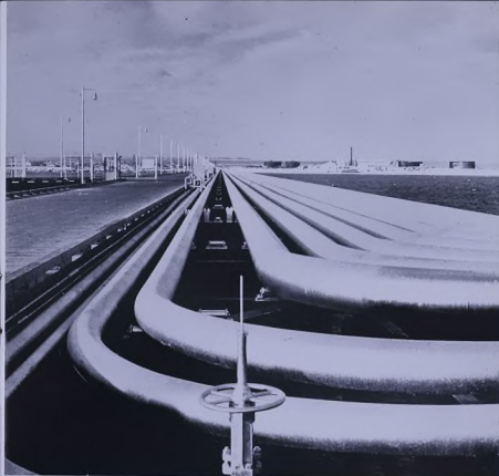
Pipeway on the oil pier
