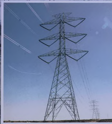
380 KV Transmission Line
