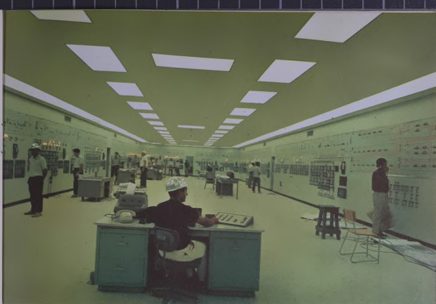
Control Room at Shuaiba Refinery
