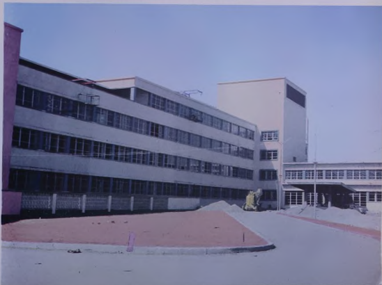
The construction of the Reza Shah the Great Hospital, in the south of Tehran, is another Plan Organization project. When commissioned, the hospital will be run by Iran's Red Lion and Sun Society.
