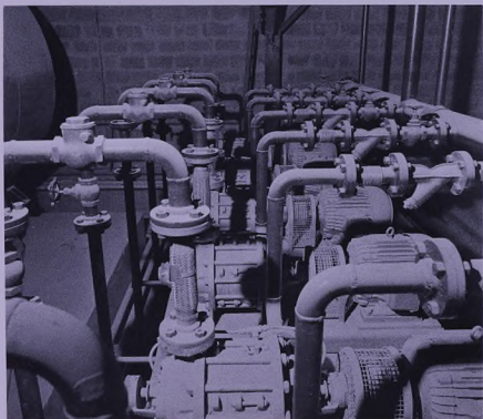
Steam boiler feed pumps
