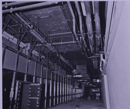
Main Corridor services
