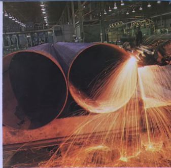
In the Ahwaz Pipe Mills.
