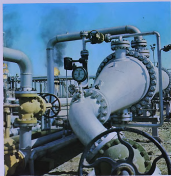
Gas-oil separator unit at Marun.
