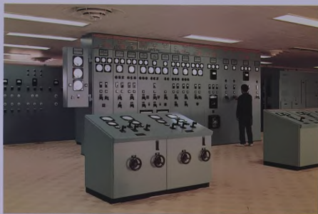
The control room at Burgan Power Station
