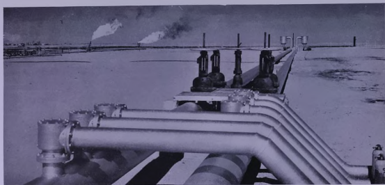
Relief valves at No.1 Degassing Station, Zubair
