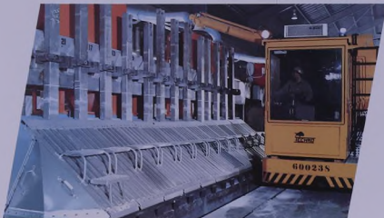
Alumina is fed to one of two hoppers mounted on each pot. Feeding is subsequently controlled by micro-processor enabling the alumina concentration to remain constant.
