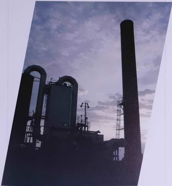
Emissions from the anode baking kilns are now 98 per cent cleaner following the installation of a new flue gas cleaning plant.
