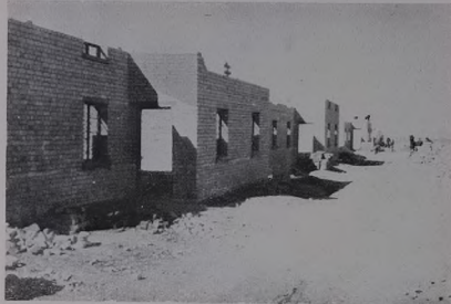
Houses under construction: top, for monthly paid workers; bottom, for daily paid workers
