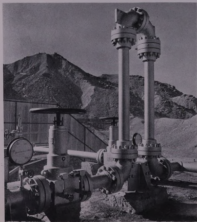
Automatic flow valve at Agha Jari
