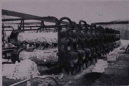
Heat Exchangers at the Agha Jari production unit
