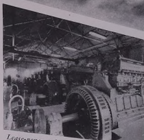
Lease-generated power station, with six 625 kva, 2400-volt, 3-phase, 60 cycle, 400 rpm generators.
