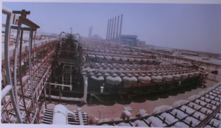
AL-JUBAIL Desalination Plant
