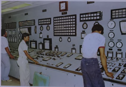
Control Room (Training in progress)
