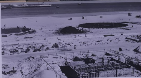
A new plant under construction at Ras Tanura will prepare refrigerated LPG for export on tankers.
