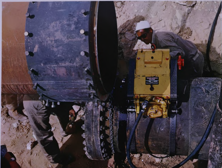
Workers connect the main links of the new pipeline to the southern part of the Ghawar field.
