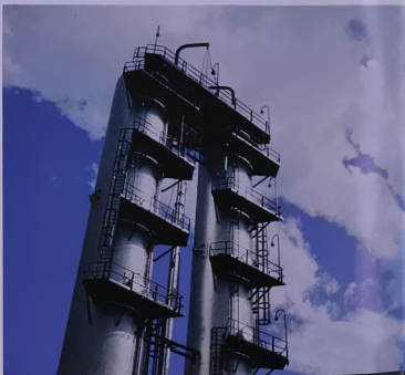
At Kirkuk No 10 Unit was added to the Process Plant in 1957
