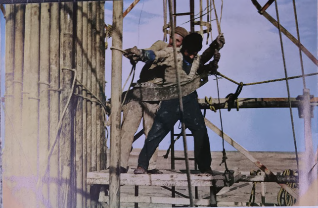
LEFT Handling a stand of drill pipe on Rig No 5 at Injana
