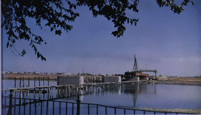
Construction of the ID 750,000 dual carriage-way bridge over the Tigris at Mosul
