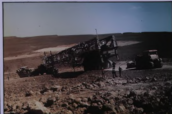
This photograph which was taken in Fahud by toolpusher, Jerry Klinkhamer, shows how bulldozers are used to prevent the rig from running away down a hill during a rig move.
