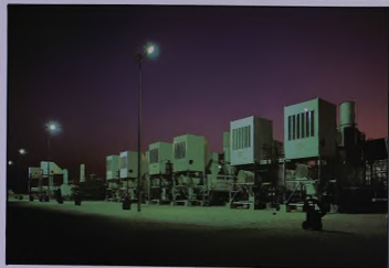
The turbines of the NGL plant at Yibal keep on turning throughout the night.
