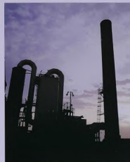
The kilns flue gas cleaning plant
