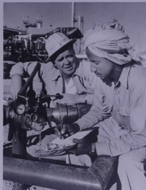
Fire experts James V. Westling and Muhammad ibn Hazza' check hydrant pressure at Ras Tanura.
