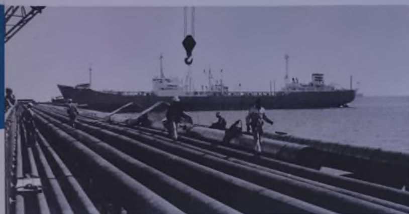
New pipelines at north pier of Ras Tanura terminal increase Aramco's capacity for loading tankers.
