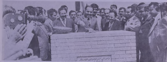
Mr. Taha Jarzawi, member of the Regional Leadership of the ABSF, Minister of Industry and Minerals, laying the foundation stone of the phosphate mines in Akkashat
