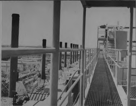
A part of the power and water distillation plant
