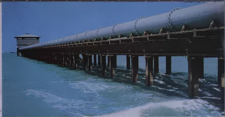
A pumping station and a Jetty of the distillation plant
