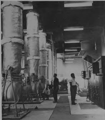
Electric generators and water pumps at Al - Raudhatain station
